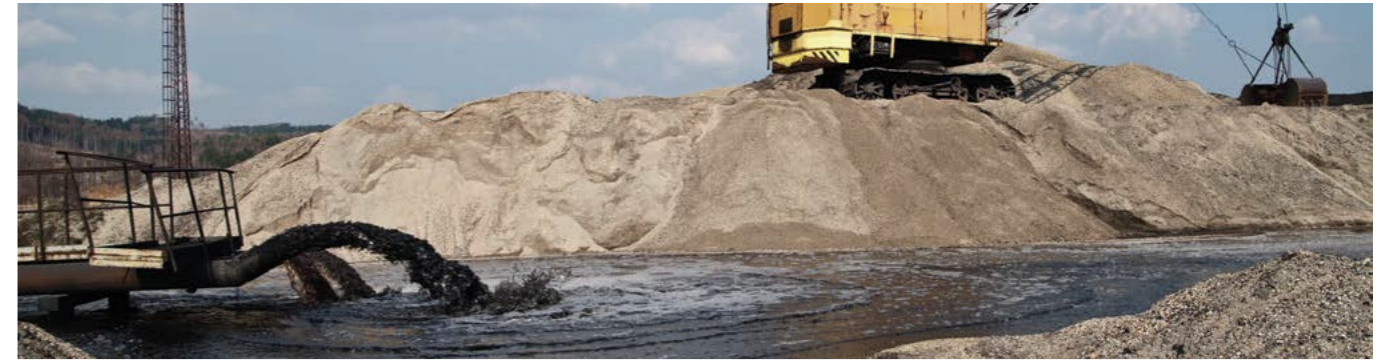
Heavily Contaminated Sludge Treatment
